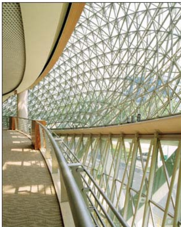
The glazing within the structural grid of the domes features triangular panes of 29mm-thick insulating glass.
